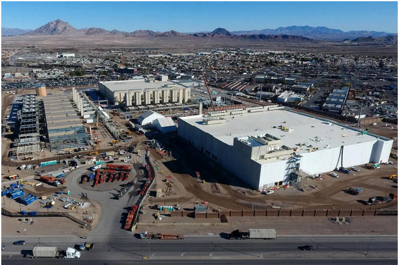
A data center under construction in Henderson. Image from the Las Vegas Review-Journal .
